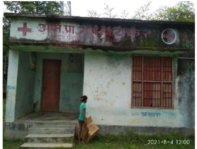
Inadequate infrastructure of PHC Building Binodpur, Madhubani
