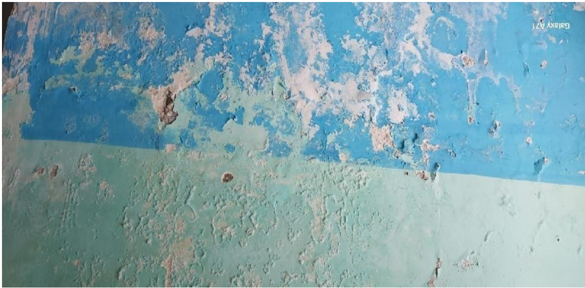
The condition of the CHC building is not good because of Seepage issue
