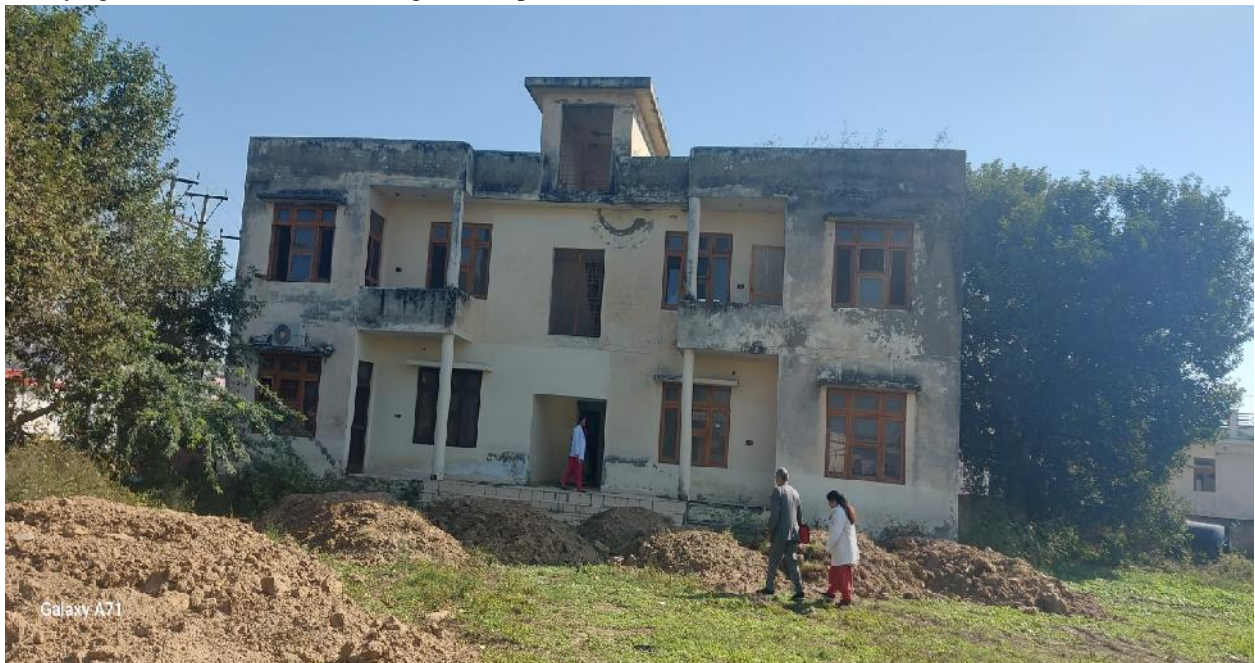
Newly constructed building with construction faults
