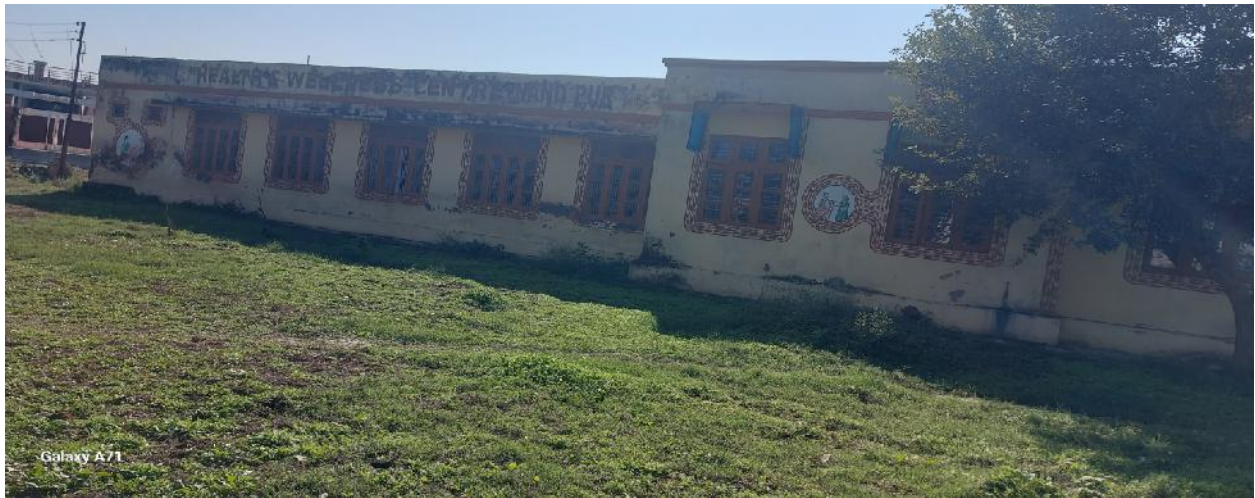
Low lying area of PHC's main building of Nandpur
