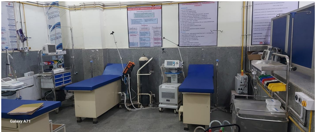
Fully Equipment of Emergency Room at CHC Banihal of District Ramban
