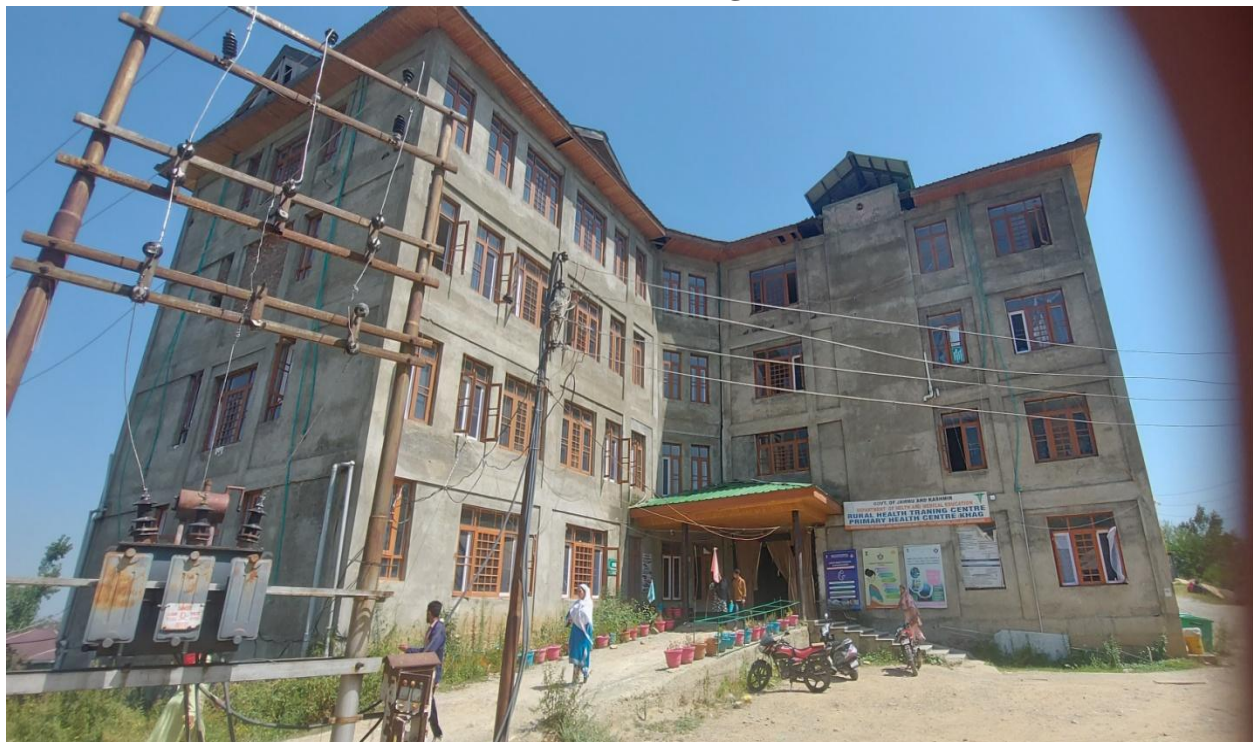
Under construction building of PHC Khag which has been constructed GMC Srinagar
