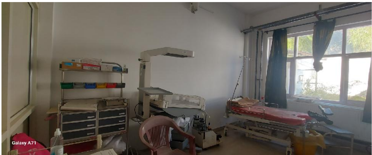
Labour Room at CHC Atholi is not in good conditions
